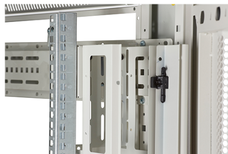
High-density vertical cable management
