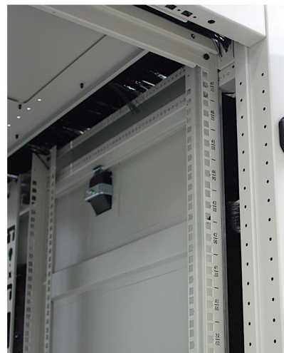
Airflow Management Baffles
