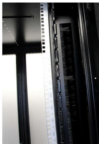
Airflow Management Baffles
