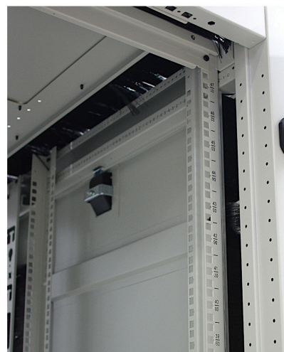
Airflow Management Baffles
