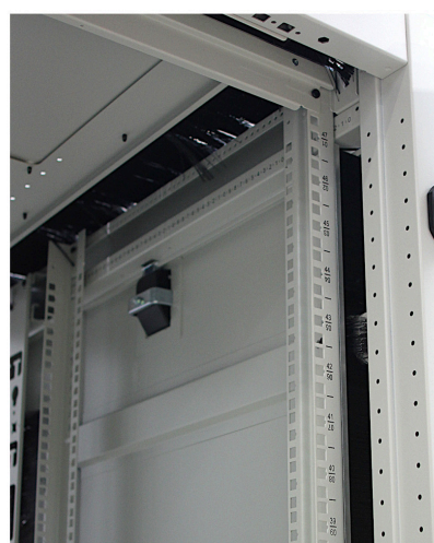
Airflow Management Baffles
