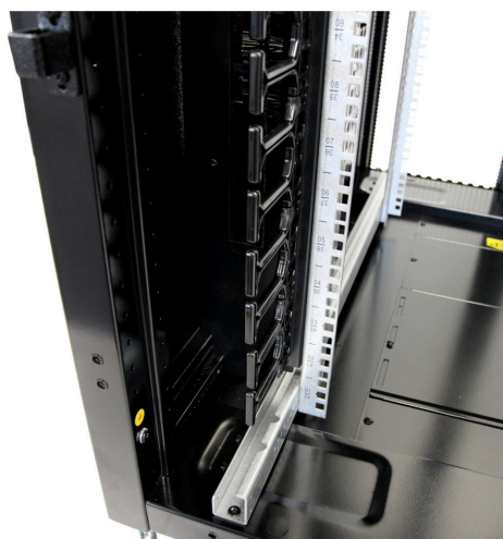
Front Finger Cable Management
