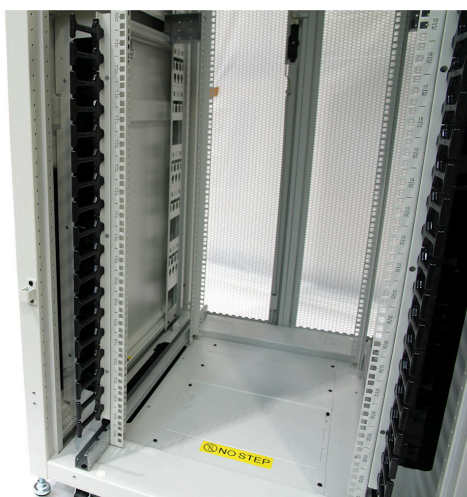
Front Finger Cable Management
