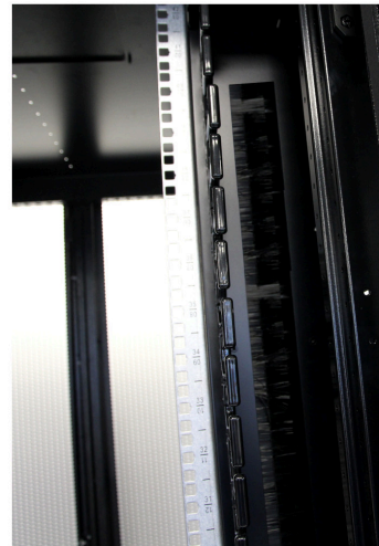
Airflow Management Baffles
