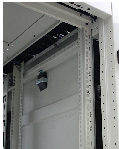
Airflow Management Baffles
