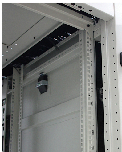
Airflow Management Baffles
