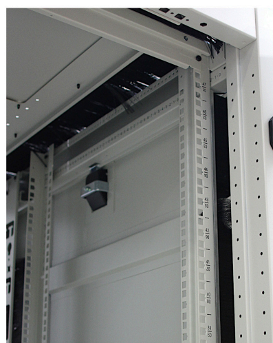
Airflow Management Baffles
