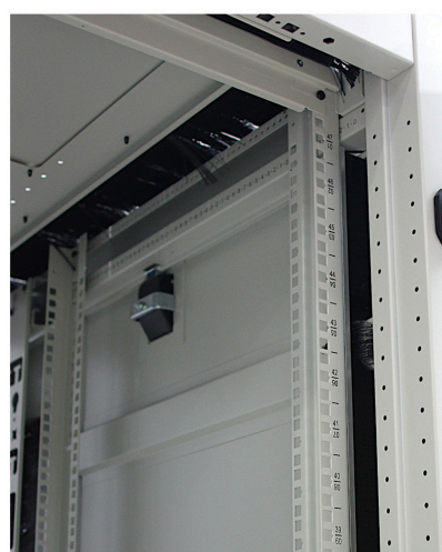
Airflow Management Baffles
