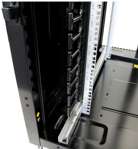
Front Finger Cable Management
