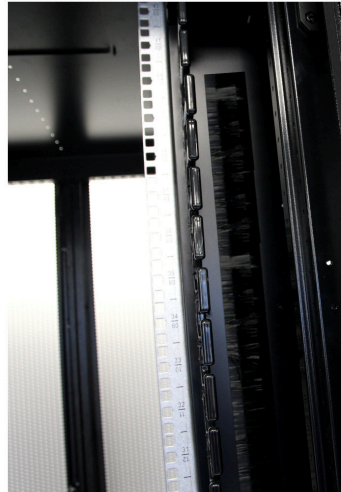
Airflow Management Baffles
