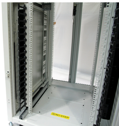
Front Finger Cable Management
