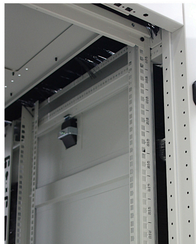
Airflow Management Baffles
