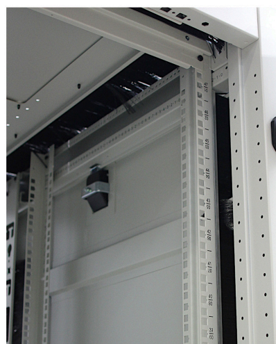
Airflow Management Baffles
