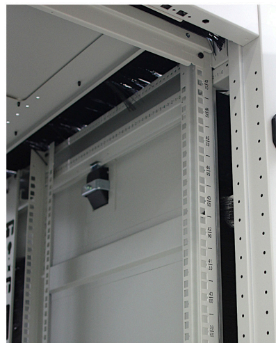
Airflow Management Baffles
