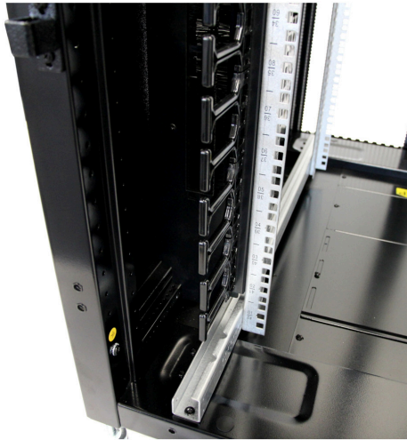
Front Finger Cable Management
