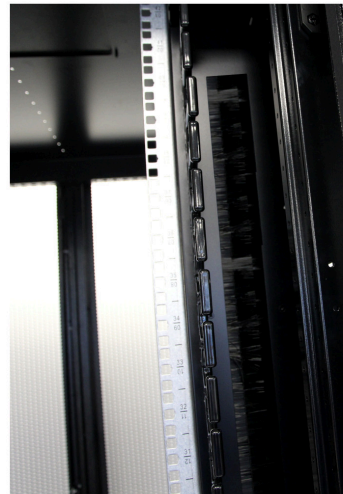
Airflow Management Baffles
