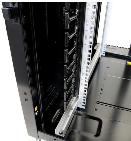
Front Finger Cable Management
