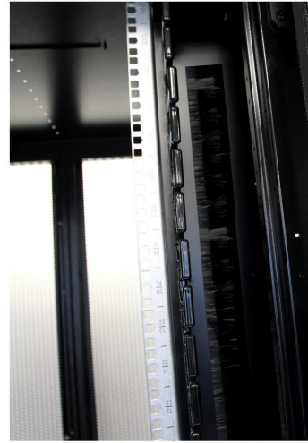
Airflow Management Baffles
