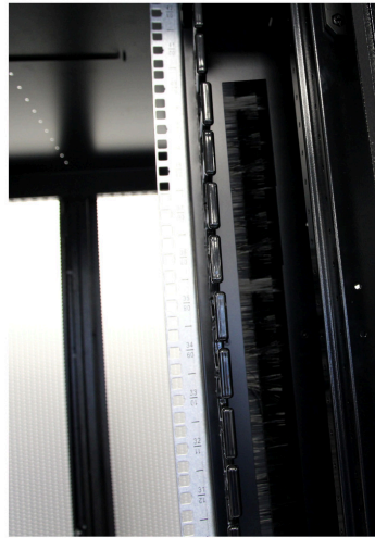
Airflow Management Baffles
