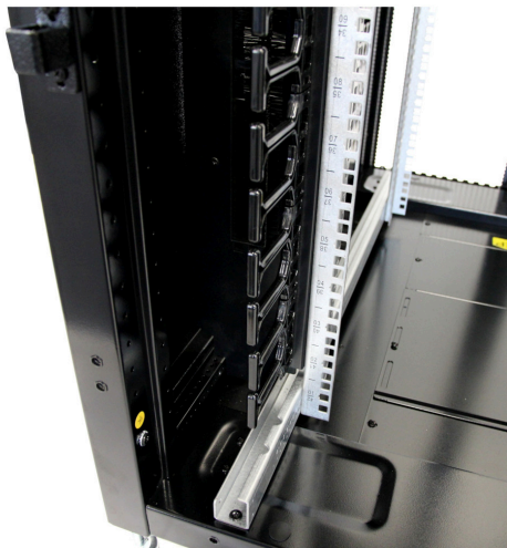
Front Finger Cable Management
