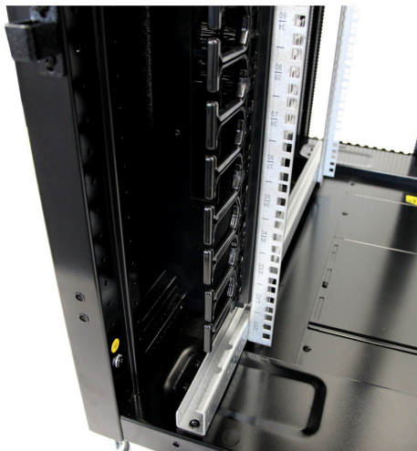
Front Finger Cable Management
