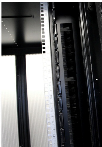
Airflow Management Baffles
