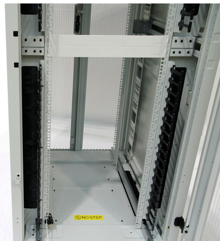
Airflow Management Baffles
