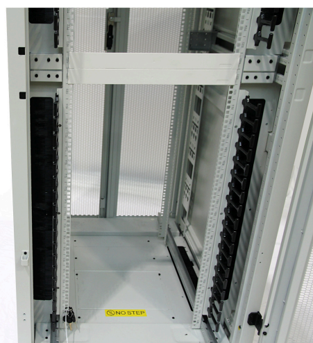
Airflow Management Baffles
