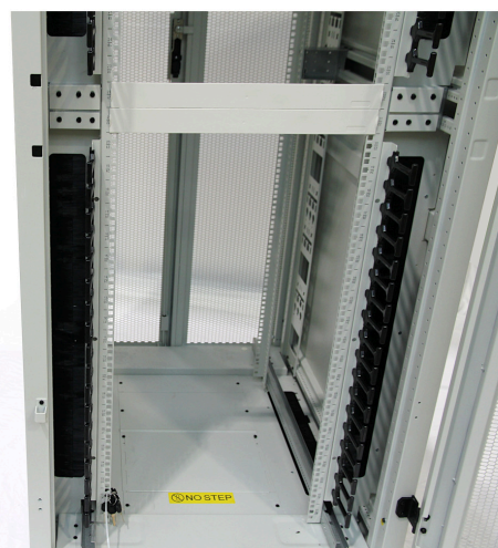
Airflow Management Baffles
